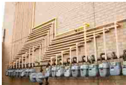
gas meters – industrial pattern
