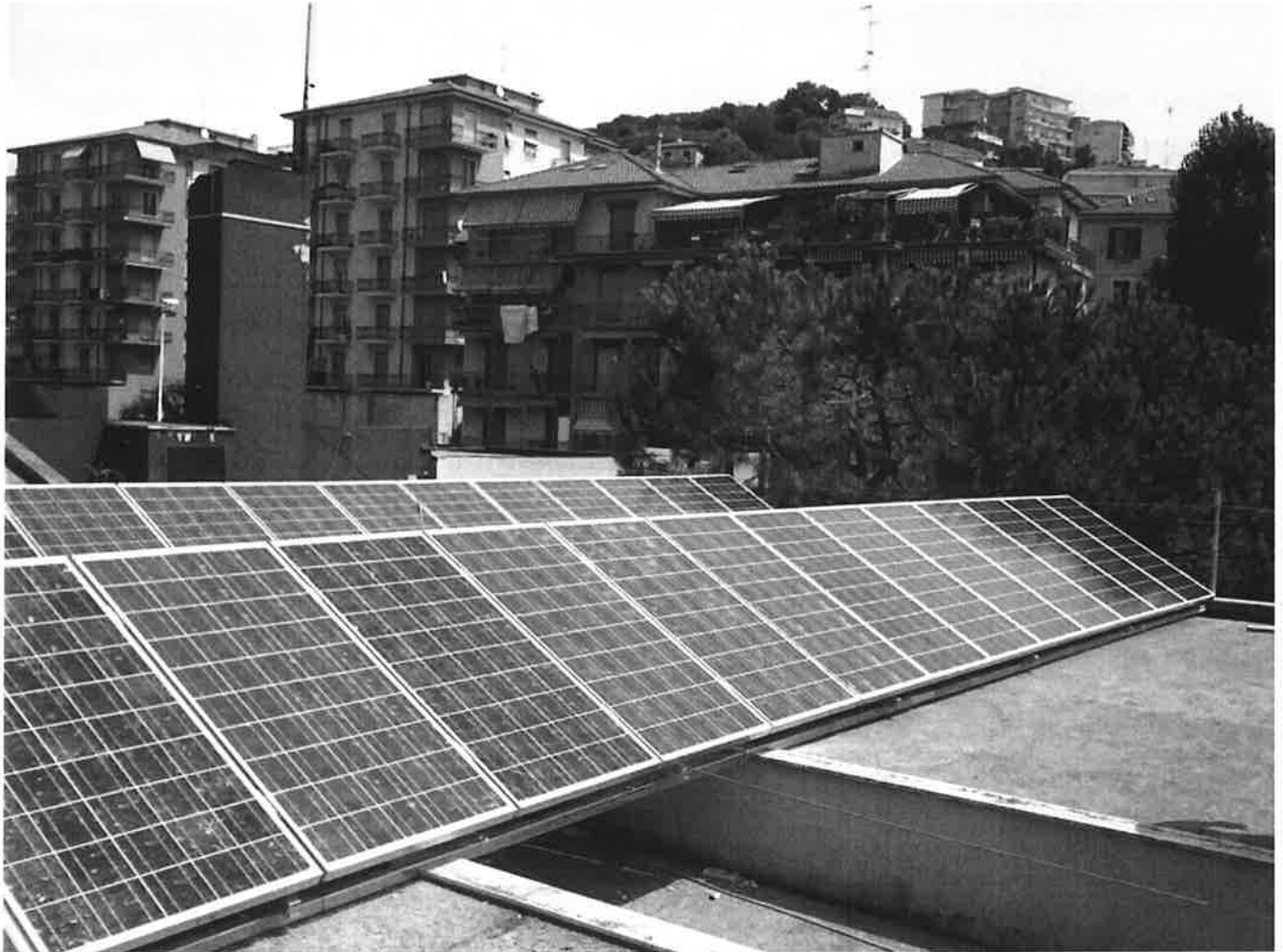
A residential PV system in Italy.
