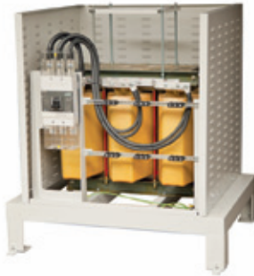
Transformer in its protection box
