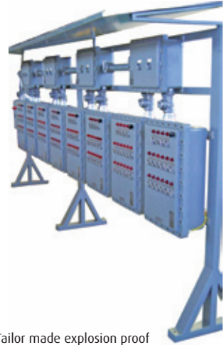
Tailor made explosion proof switchrack and panel boards
