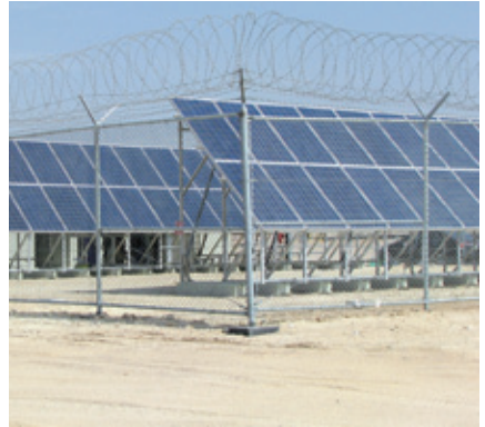
Solar off-grid power plant 15 kW 50 Vdc installed in North Kuwait on behalf of Kuwait Oil Company (KOC)
