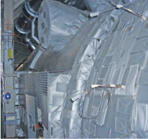
Side of a 300MW Gas Turbine
