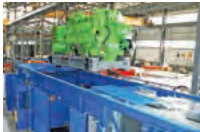
1500 kVA Medium Voltage Genset (Under Construction)
