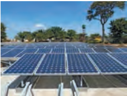
Hybrid solar/wind off-grid power plant 90 kW installed in Kashobwe, D.R. Congo
