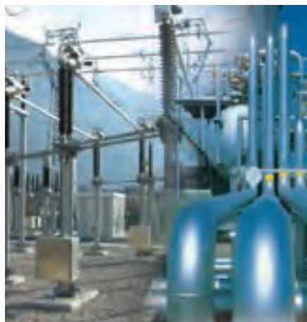
Automation and communication for utilities
