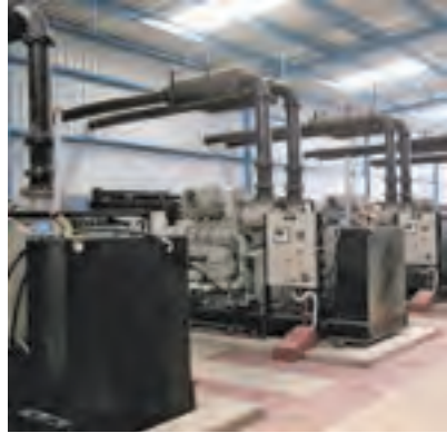
Power Generation: Oil and Gas Power Plant
