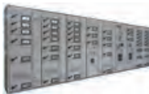
Multicontrol LV Motor control center switchboard
