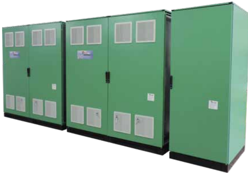
Highly customized 3-Ph industrial UPS 2x250 kVA, installed at Al Dhakhira STW plant, Qatar
