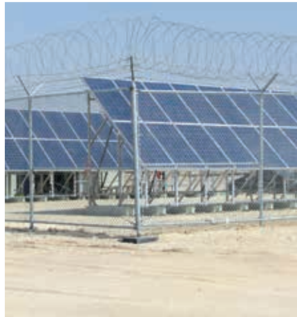
Solar off-grid power plant 15 kW 50 Vdc installed in North Kuwait on behalf of Kuwait Oil Company (KOC)
