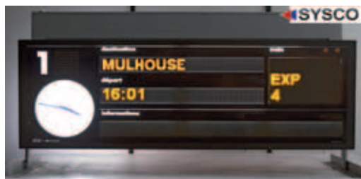
Equipment for Passenger Information Display System PIDS
