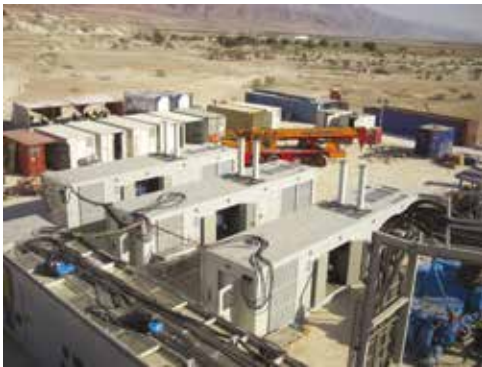
DGS for continuous power supply 24/7 for Drilling Stations with parallel operation and containers designed for desertic environmental conditions
