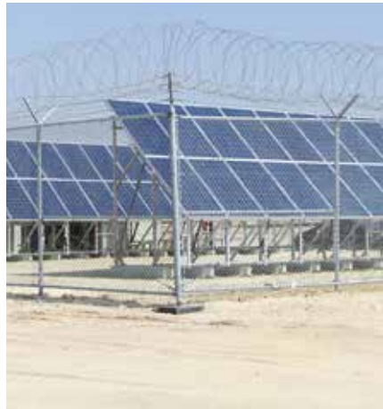
Solar off-grid power plant 15 kW 50 Vdc installed in North Kuwait on behalf of Kuwait Oil Company (KOC)
