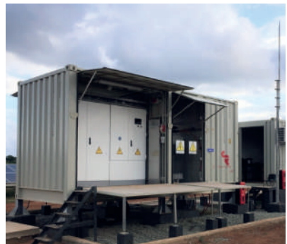
Solar Station ISO Container 1-5 MWp
