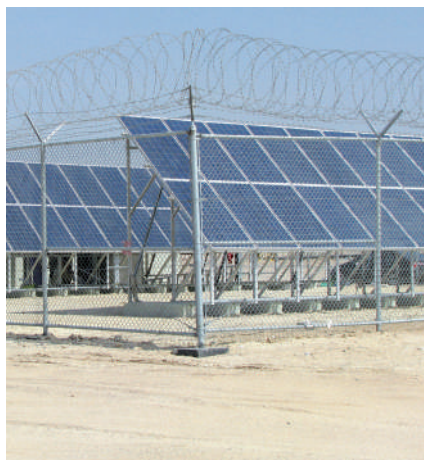
Solar off-grid power plant 15 kW 50 Vdc installed in North Kuwait on behalf of Kuwait Oil Company (KOC)
