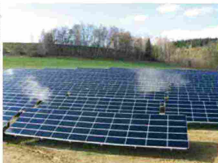
A solar PV project installed by Juwi Holding AG in Trebovice, Czech Republic.
