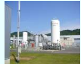
Gas cogeneration system
