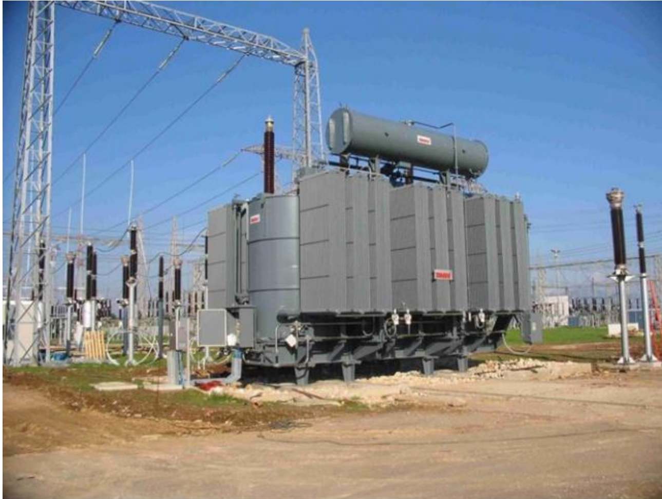
TERNA - Three-phase Shunt Reactor 200 Mvar, 400 kV
