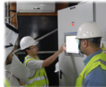
Road Lighting Control System
