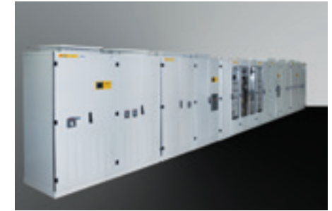
UPS system composed with two rectifiers 125Vdc 1200 A and two inverter 220Vac 1Ph output, central change over systems
