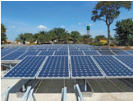
Hybrid solar/wind off-grid power plant 90 kW installed in Kashobwe, D.R. Congo
