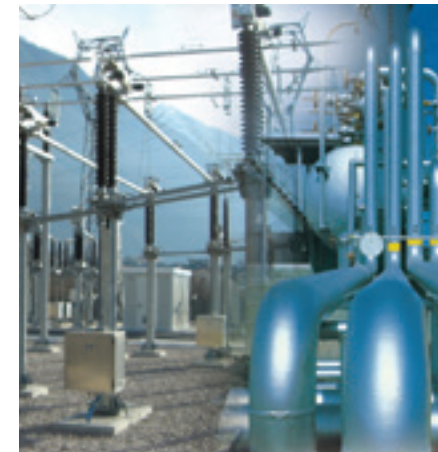
Automation and communication for utilities
