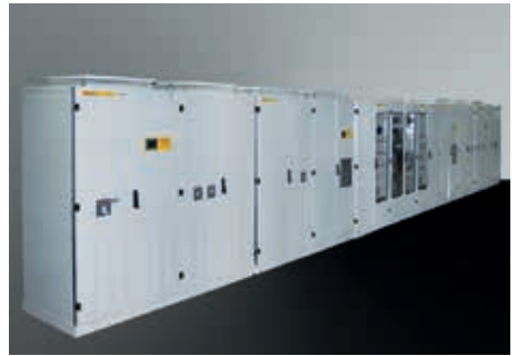
UPS system composed with two rectifiers 125Vdc 1200 A and two inverter 220Vac 1Ph output, central change over systems
