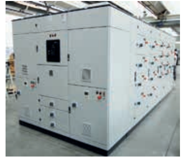
Automation and distribution metal enclosures
