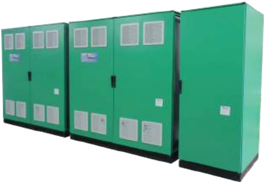
Highly customized 3-Ph industrial UPS 2x250 kVA, installed at Al Dhakhira STW plant, Qatar
