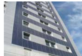
Building integrated front wall - 40KwP
