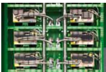
Sodium-nickel chloride battery bank installation
