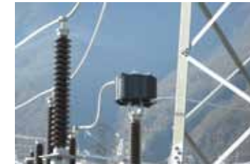
Installation of line traps
