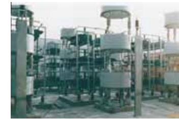
MV and HV Power Factor Correction Banks and Harmonic Filters
